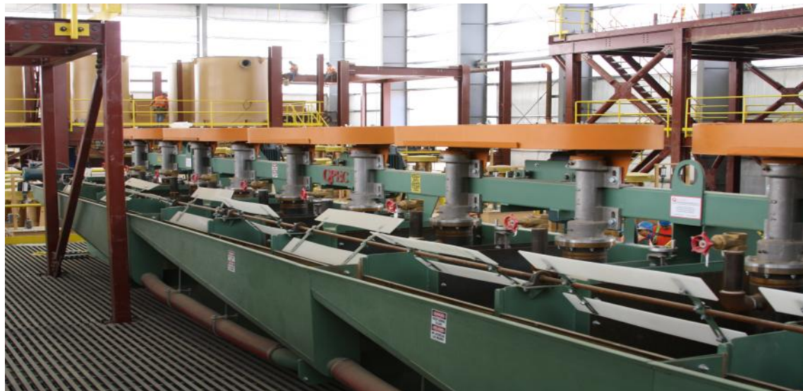
2 ea QPEC 10 Cell Banks of No. 18 Spl Flotation Machines
